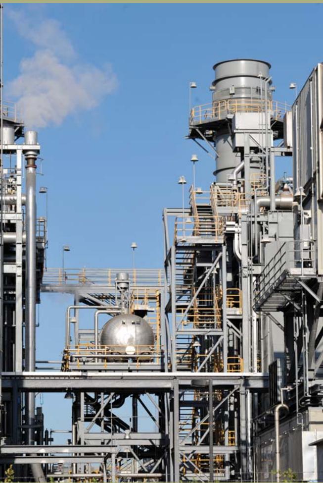
Malburg Generating Station
