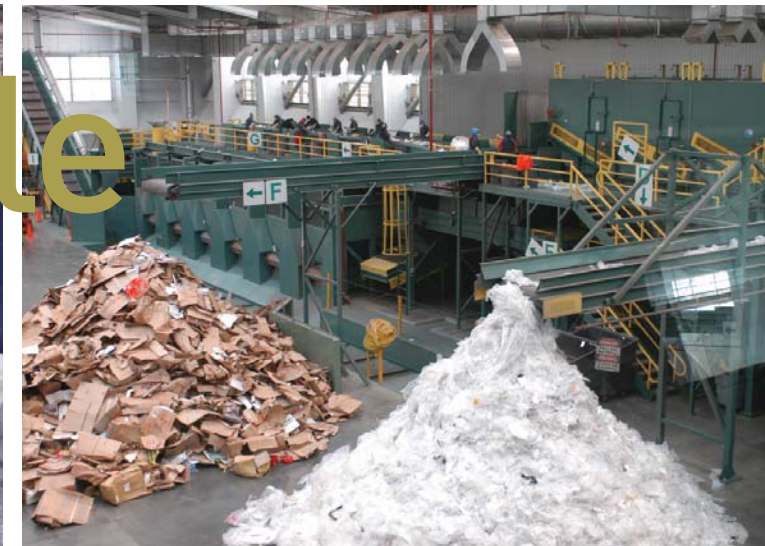
Recycled cardboard and plastic recovered at the Puente Hills material recovery facility
