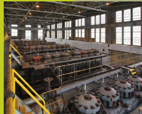
Diesel generators at the Vernon Power Plant built in the 1930s
