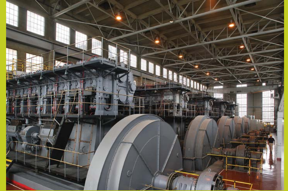
Diesel generators in the Vernon Power Plant
