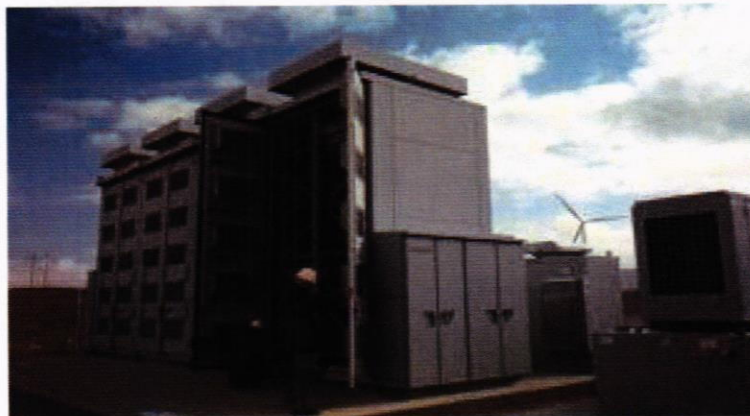
Figure 3 Lead-Acid Battery Storage
