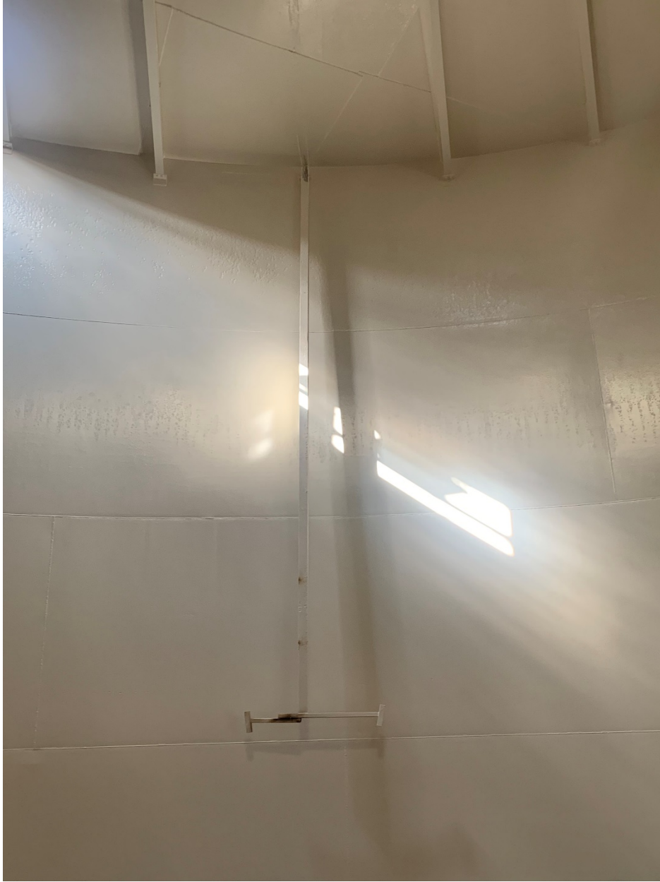
Figure 5: Failed header and jack rafter
