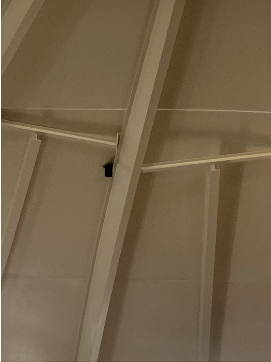
Figure 3: No mechanical connection between header and main rafter
