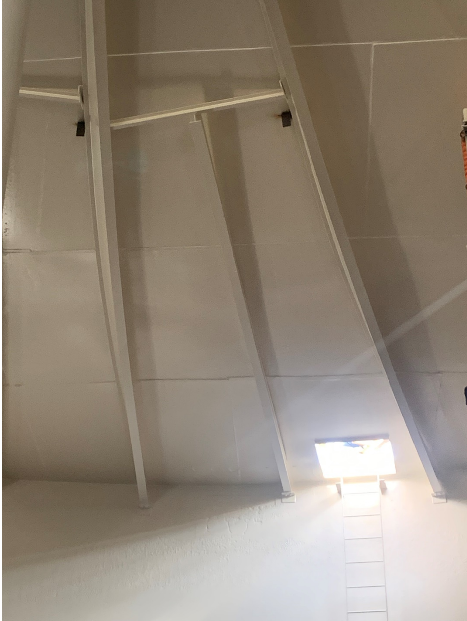
Figure 1: Twisted rafters. Partially failed header and jack rafter
