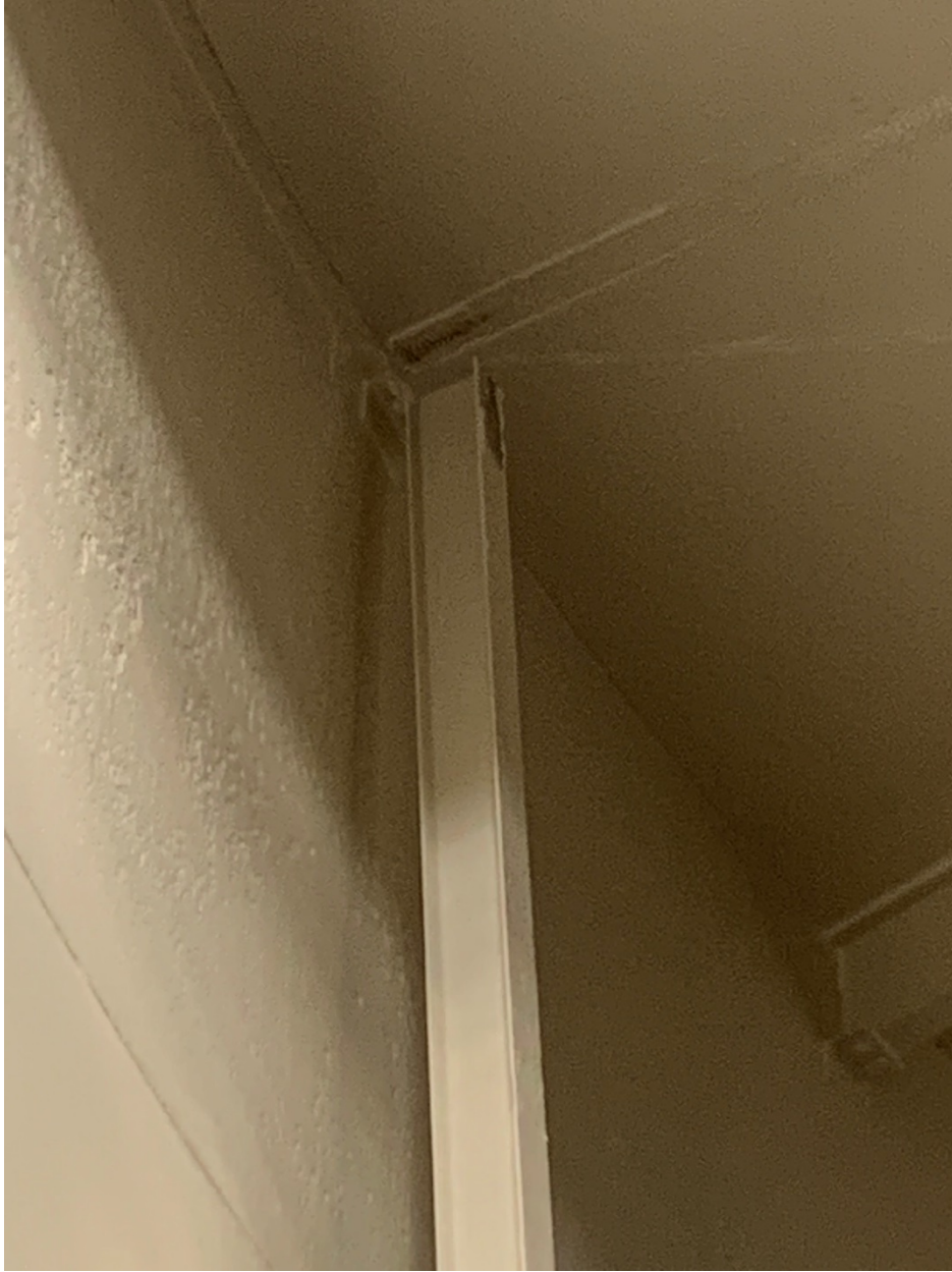
Figure 6: Shell and jack rafter connection after failure
