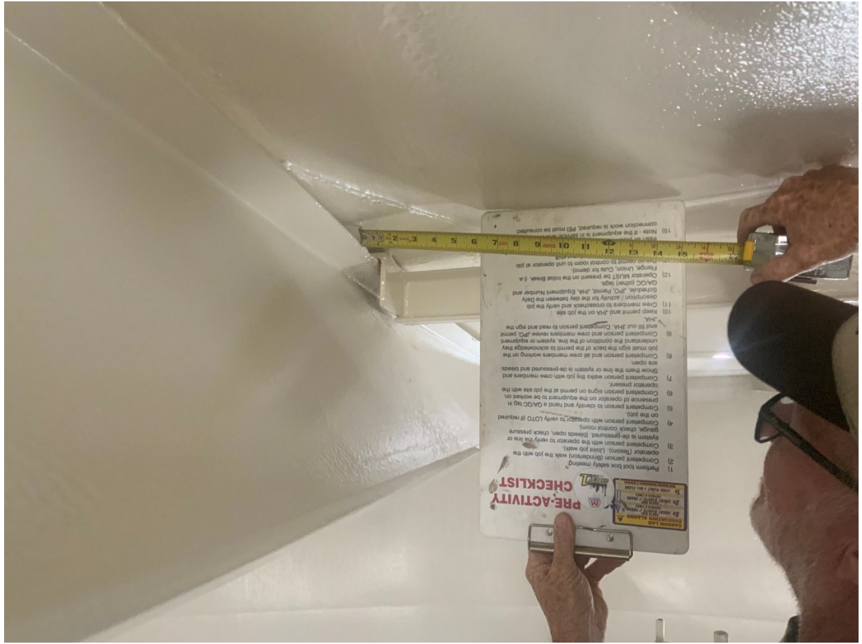
Figure 2: Close-up of twist in main rafter
